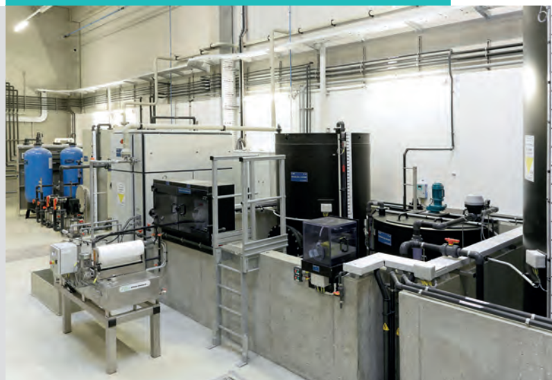
Treatment plant for liquid waste from the aeronautical industry.
